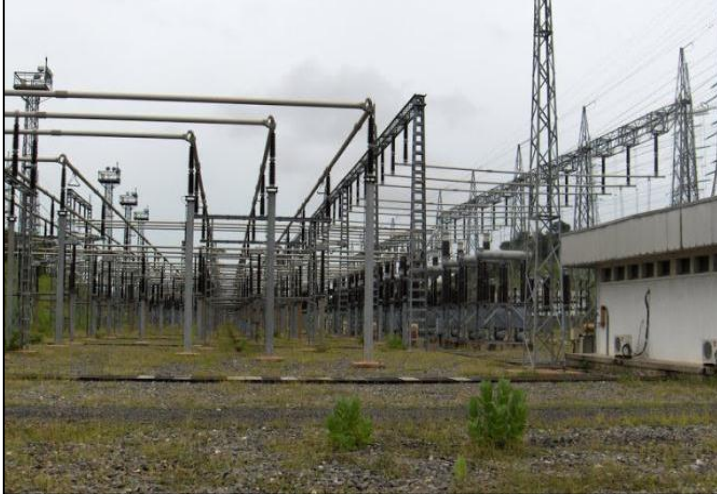
Figure 25: Poste de SADEMI/SNEL (BANDUNDU)
